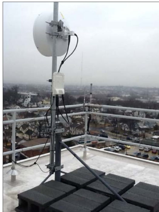
Image of PTP 650 Link, ballast weight temporary mount, roof of HackensackUMC
